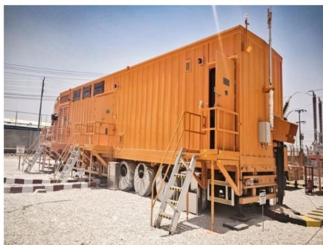
Figure 8: TGood delivered 15 units of 132kV mobile substations for National Grid SA, Saudi Arabia in 2025
