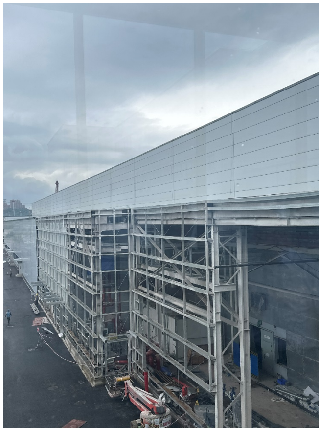
Figure 6. Chongqing Hitachi Energy's phase three capacity expansion
