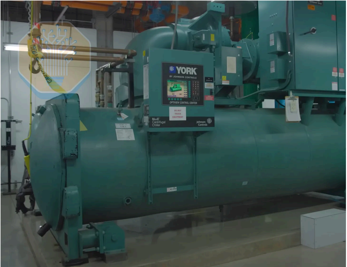
Chiller Plant at Oklahoma City Datacenter. Source: Matthew Berman
